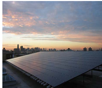
Rooftop solar array
